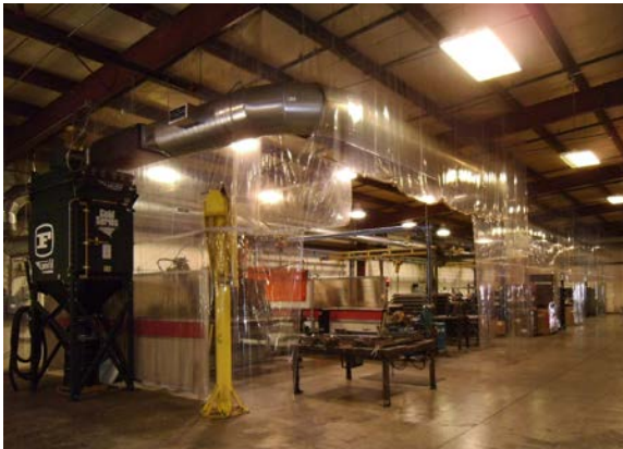
Example of a well-designed fume extraction system using high efficiency filtration, a custom ducting layout, and curtains to help contain contaminants within the process area.
