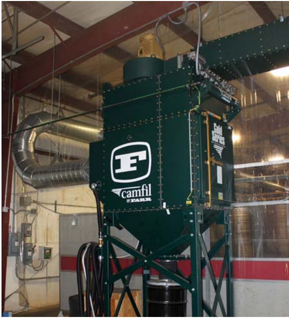
A high efficiency cartridge dust collector with top mount motor fan and silencer reduced floor space requirements and installation costs in this welding shop.
