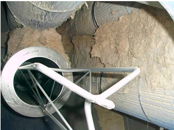
Entrained dust on horizontal filters can shorten filter life and provide a dusty surface for sparks to ignite.
