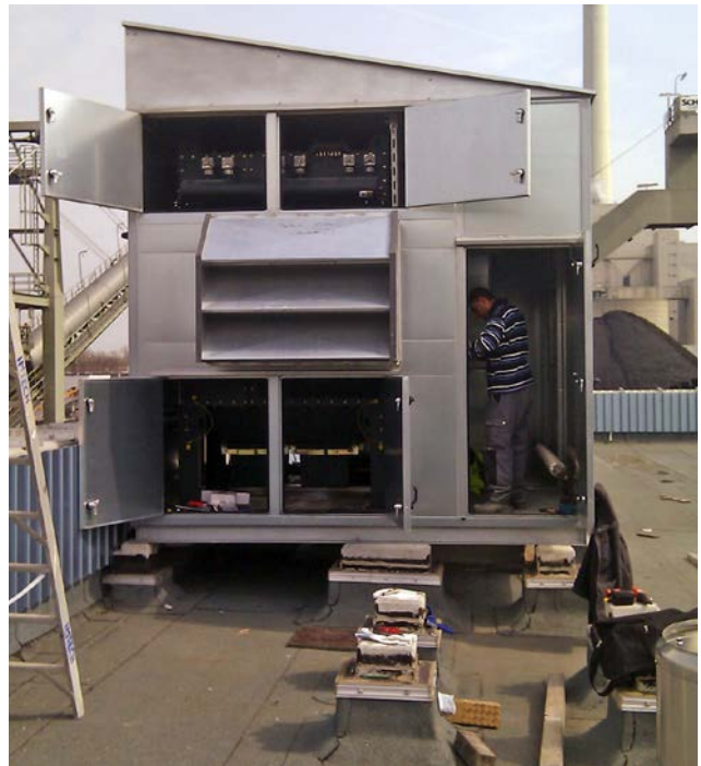
A cartridge dust collection pressurizing system is installed on the roof of a maintenance building in the harbor of a European coal power plant to prevent ambient coal dust from entering the building. The unit is installed in front of a ventilation system and uses a water and moisture eliminator filter at the intake to keep rain from entering the unit.
