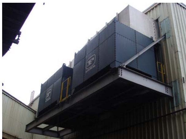
A large 24-cartridge collector plays a critical role in pressurizing an MCC room at a U.S. iron mine, protecting the electronic equipment from possible short circuits created by dust infiltration.
