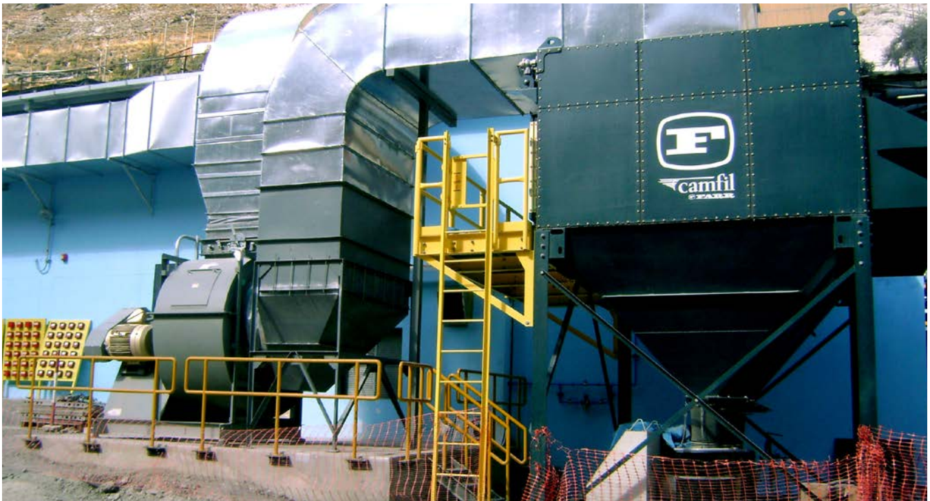
Working at a 15,000+ ft. elevation, this 48-cartridge dust collector pressurizes and conditions the control room of a gold and silver mine.
