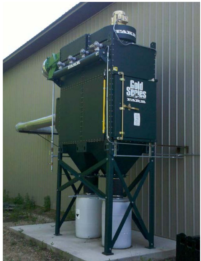
Eight-cartridge dust collector captures laser cutting fumes from an automated tube cutting application.
