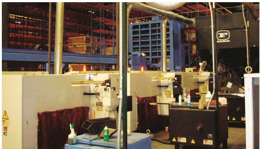
A collector with 20 filter cartridges, shown in back right, captures dust and fumes from three laser tables at an engine manufacturing facility.
