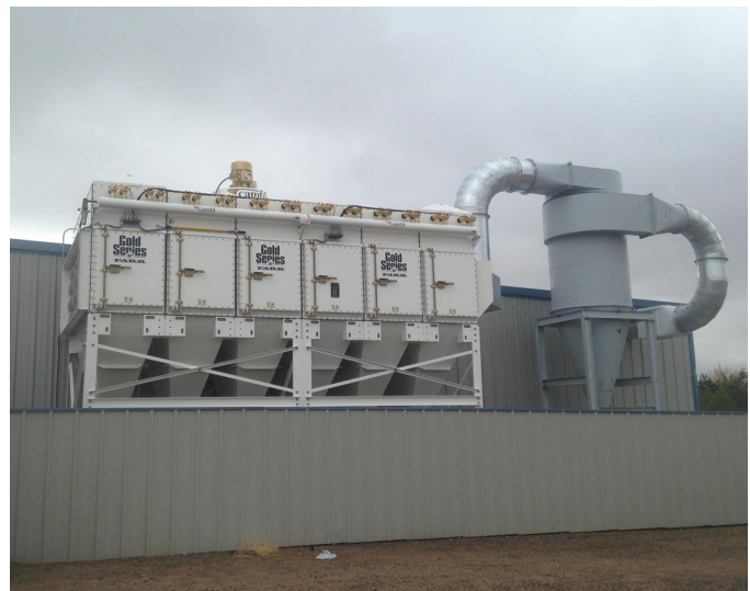
Dust collector serving a twin wire arc application uses 72 high-efficiency filter cartridges and a cyclone pre-separator that enhances cleaning efficiency and acts as a spark arrestor.
