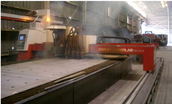
Before the Farr Gold Series® collector was installed smoke from plasma cutting operation filled the facility.
