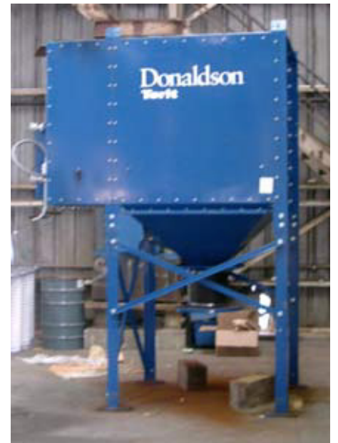
The problem Torit dust collector.
